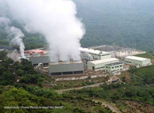
Fig. 8: Geothermal Plant of Berlin, El Salvador. Configuration: 2 X 30 MW, 1 X 35 MW.
